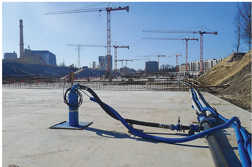
Figure 3 Well head and discharge pipe for a deepwell dewatering system for an open cut excavation (courtesy WJ Groundwater Limited)
