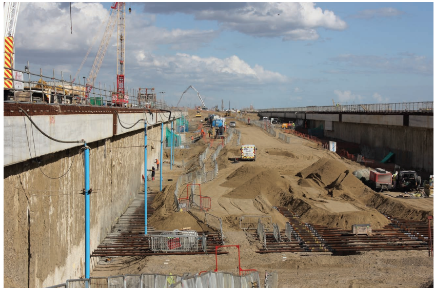
Figure 2 Deepwell dewatering for groundwater control for a large excavation within retaining walls (courtesy WJ Groundwater Limited)
